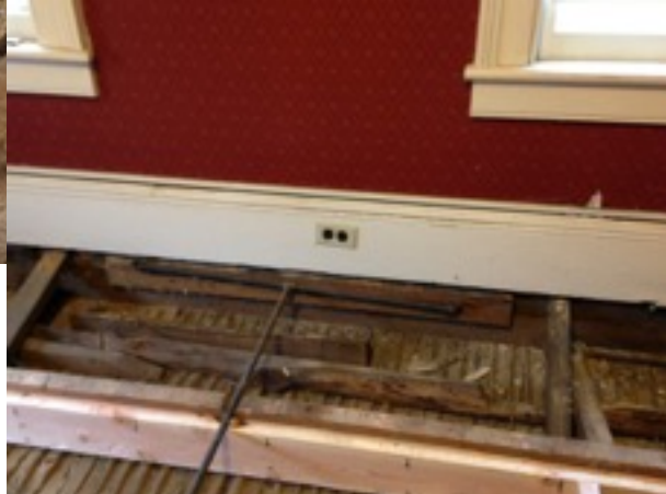
Sistering joists in conference room (above) and office (left) where an old gas pipe T junction under the floor remains a mystery.
